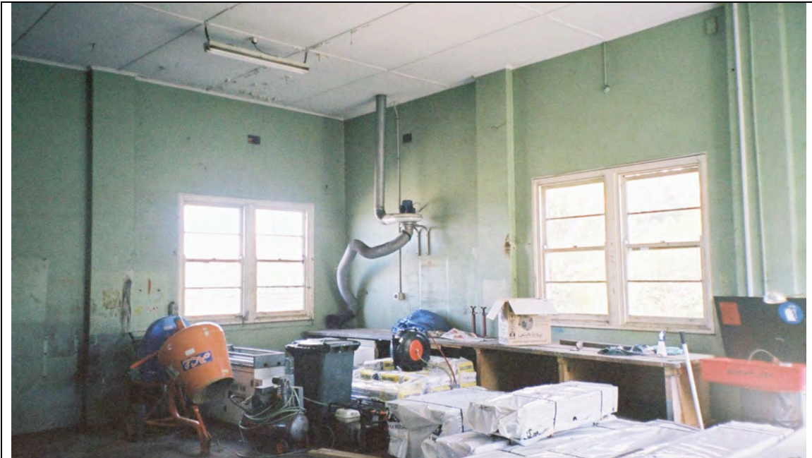
Current view of interior of west room of Building 6 (Photo: Robertson & Hindmarsh Pty Ltd, 2006)
